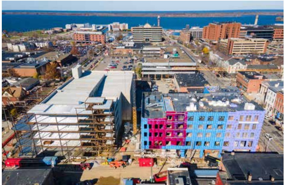
This aerial view of the new construction happening along West 5th Street between State and Peach shows a glimpse of the massive scope of work being completed by the EDDC. / Corey Cook
