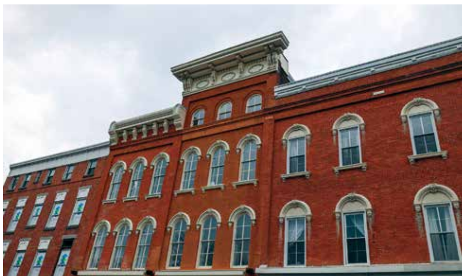
The buildings lining North Park Row's western block have all recieved a large amount of structural preservation work at the hands of the Erie Downtown Development Corporation, ensuring they stand tall for generations to come. / Jessica Hunter Photos
